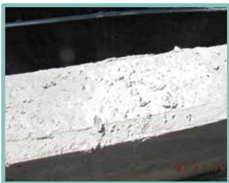
▲ 擋土牆澆置後未鏟平不平整
