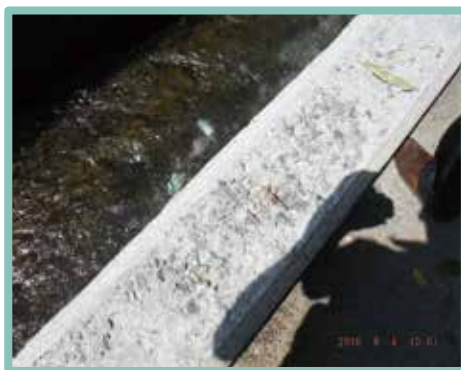
▲ 擋土牆澆置後未鏟平不平整
