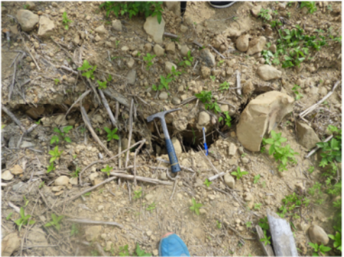
10.崩崖裂隙 (E=207802.13, N=2598870.74)
