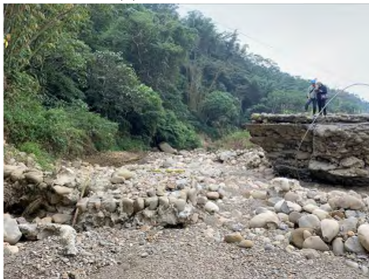
(c) 副壩左側毀損
