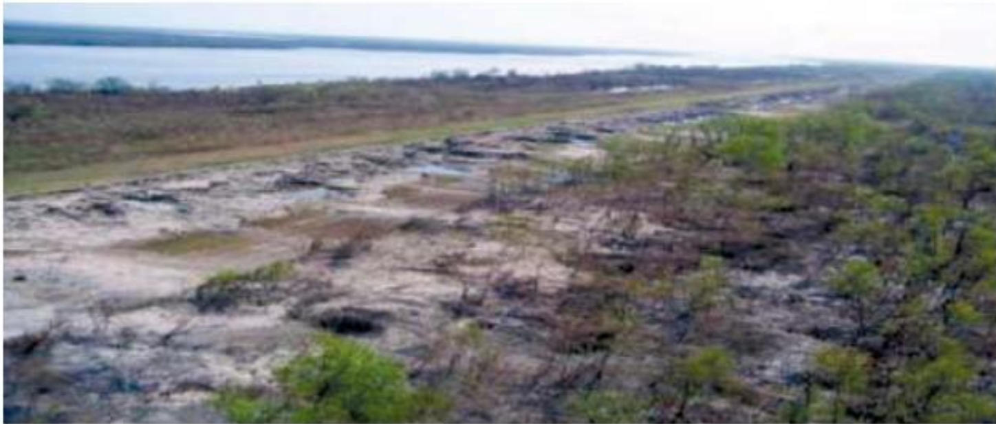
Figure 7.12 Obliterated Levee along the Mississippi River-Gulf Outlet
