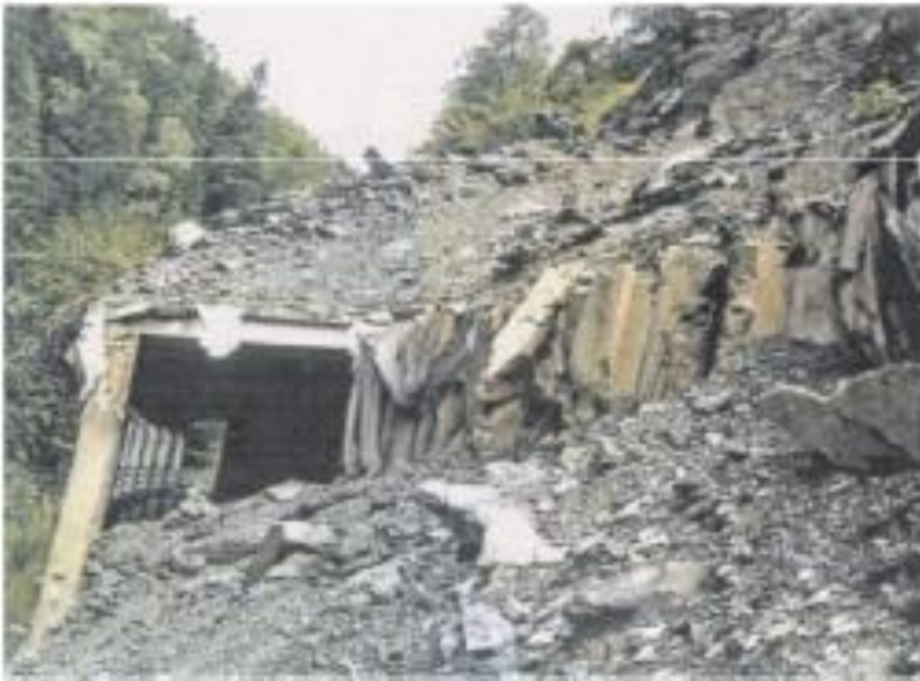
Figure 88. Concrete shelter damaged by heavy rockfall
