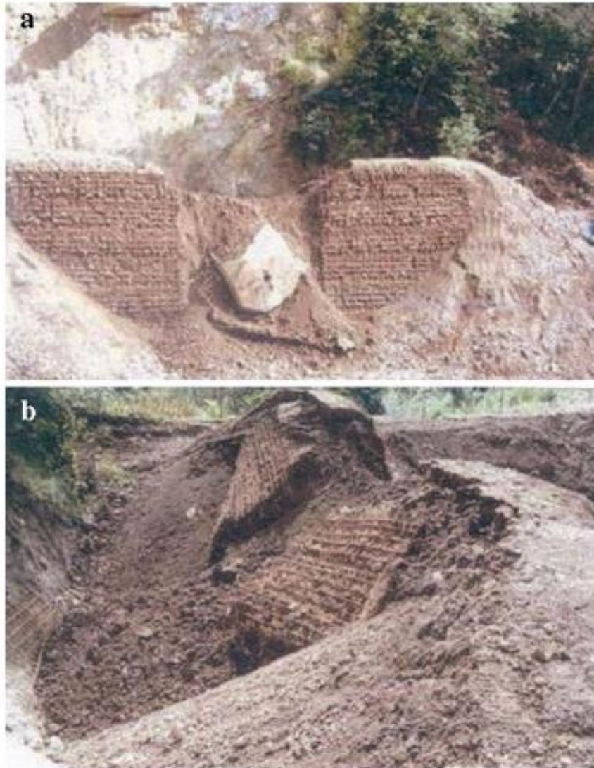
Collapse of unreinforced soil barrier
