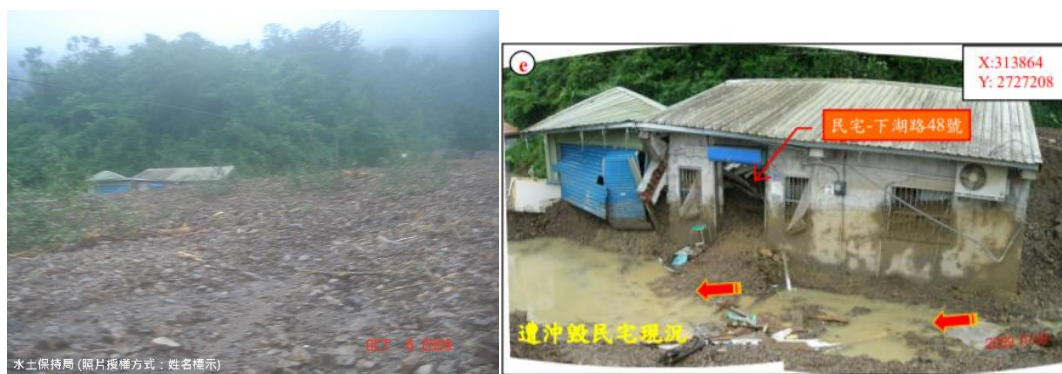
(a) DF135 房舍淤積全景(2009/10/06) (b)房舍淤積近照(2009/10/09)
