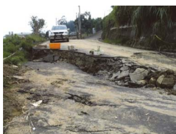
滑動破壞使道路沉陷 Road subsidence due to sliding failure of hillside
