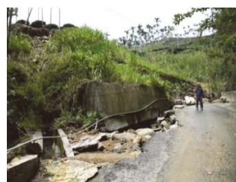
主要道路旁之擋土牆損壞 Damage of retaining wall beside main road
