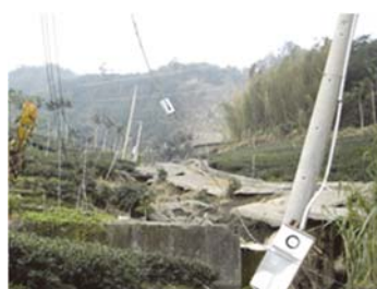
擋土牆損壞使道路沉陷 Road subsidence due to damage of retaining wall
